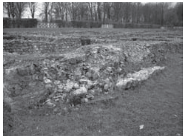
Figure 4. Present bad state of conservation in a public bath (2008), excavated and restored 50 years ago in the Civilian town in Petronell-Carnuntum (Franz Humer, Haslau a.d. Donau).
