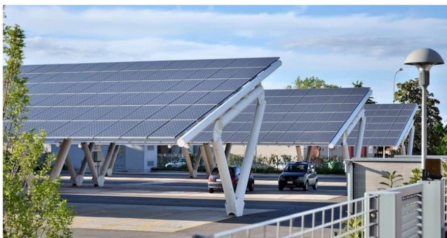
Figure 3: Solar canopies installed in parking lots [48].
